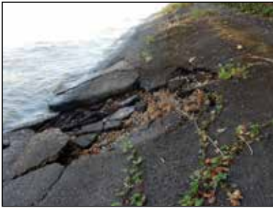
Deteriorating Revetment at Perkins Peninsula County Park
